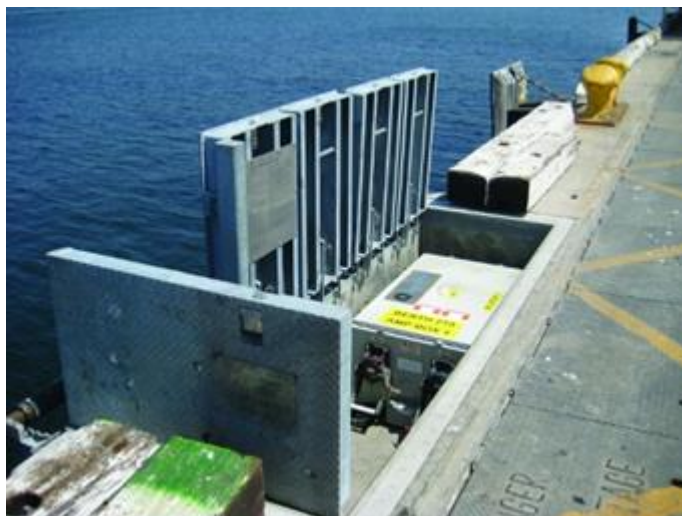
Slika 9: Sistem AMOVault, proizvajalec Cavotec; Vir: spletna stran https://www.cavotec.com/en/your-applications/ports-maritime/shore-power/shore-power-systems-for-ports
